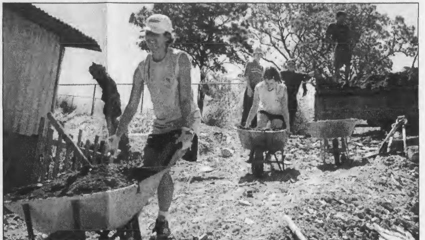
HAULIN' DIRT —Sophomore Ashley Cooper, left, and junior Sarah Rutherford, right, work on a housing expansion project in Proyecto Cristal, a shantytown in Costa Rica. Twenty-four Susquehanna students and faculty members took the trip to Central America over winter break.
